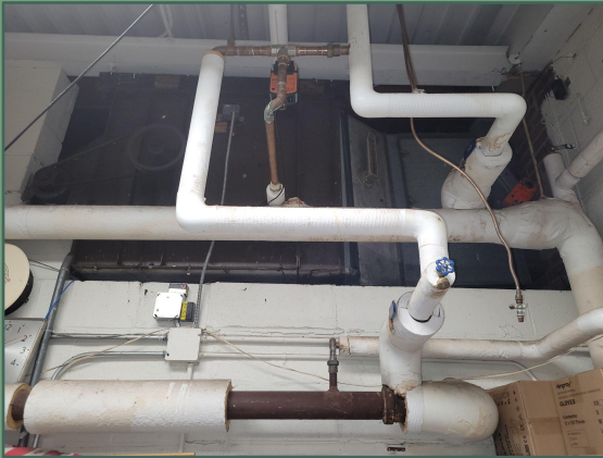
Air Handler - Gym - 1978
