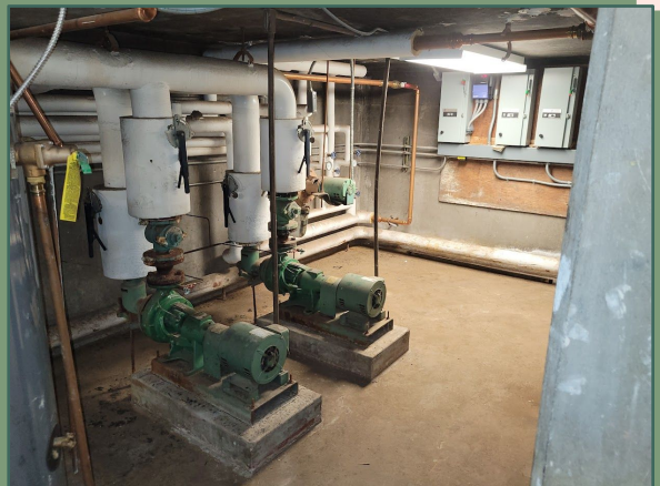
Heat Pumps & Piping - 1989
