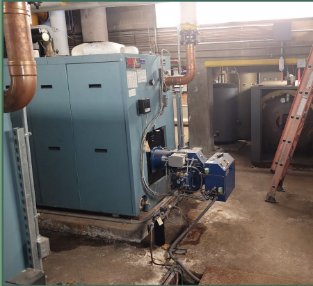
Boiler Room (2018 Boilers) - Room Always Wet Due to Groundwater
