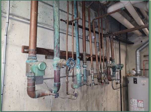
Original Water Pipes - 1949
