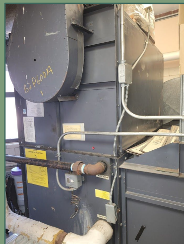
Cafeteria Air Handler 1985
