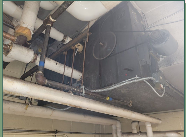
CNH Cafeteria Air Handler - 1968
