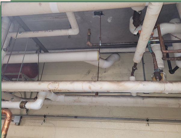
CNH Original Piping - 1968
