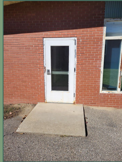
Exterior Doors 1989 Rusting at Base
