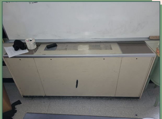
CNH/CHS Original Unit Ventilators - 1968
